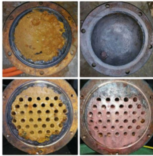
Fig. 6. Photo fouling During Commissioning (Overhaul) Earlier
