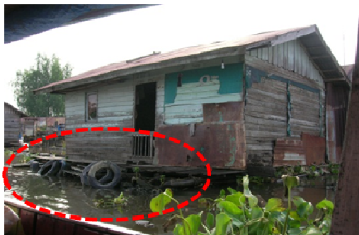
Figure 8. Semi-Fix element in the past condition. Semi-fix elements as additional elements to building frontage used tires arrangement near river-facing foundation construction
