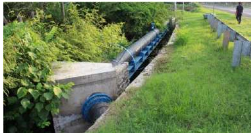
Gambar 5. Pipa transmisi SPAM Regional Kab. Gianyar, Bali (Sumber : Prasarana dan Sarana Air Minum, 2015)
