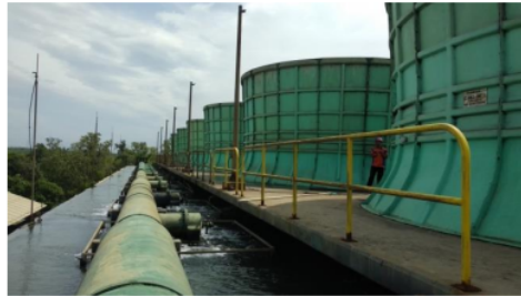
Gambar 1. Cooling Tower Unit 1 & 2 PLTU Asam Asam
