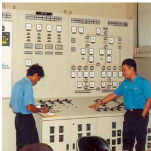
Gambar 25. Control room IPA Pejompong
