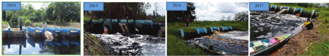
FIGURE 3. (a) Concrete canal blocking in canal E in 2014 [15], (b), (c), (d) canal blocking condition in 2015 to 2017
