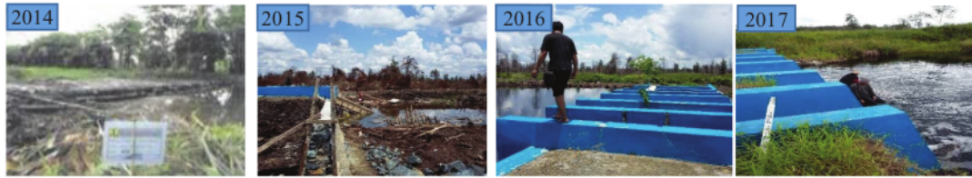
FIGURE 2. (a) Compacted canal blocking in canal D, [15], (b) redesign canal blocking in 2015, (c) canal blocking in 2016 and (d) canal blocking in 2017
