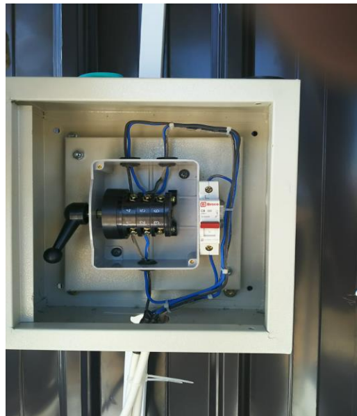
Gambar 8 Instalasi Box Panel
