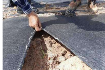
Figure 4.13 The Damage of Geotextile Joints
