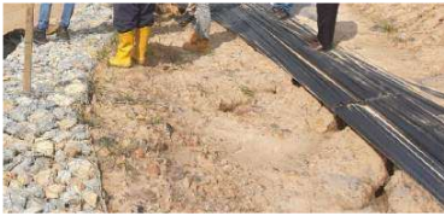
Figure 4. 14 Formation of a Natural Piping Hole Due to Water Flows from the Ground
