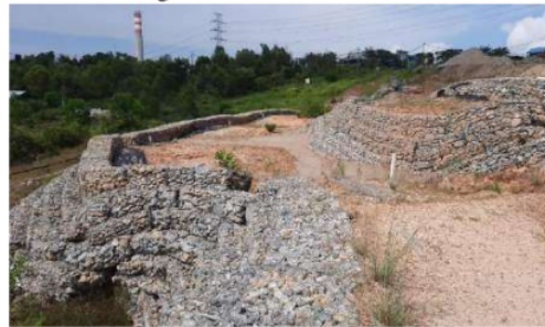
Figure 4.12 Deformation of Gabion Construction Form
