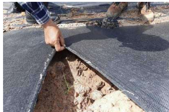
Figure 4.13 The Damage of Geotextile Joints
