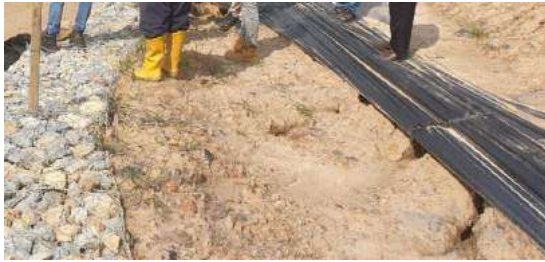
Figure 4. 14 Formation of a Natural Piping Hole Due to Water Flows from the Ground
