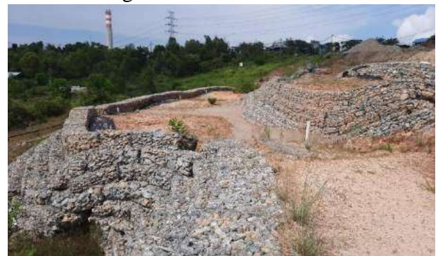
Figure 4.12 Deformation of Gabion Construction Form
