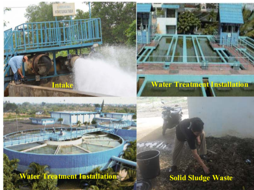
Figure 1. Water Treatment Installation 2 PDAM Bandarmasih and Solid Sludge Waste
