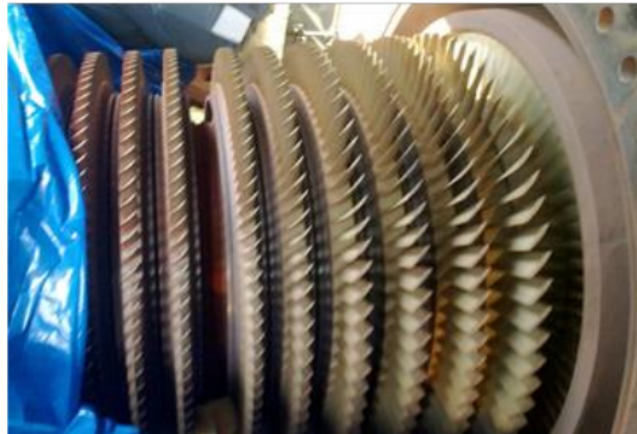
Gambar 4. Compressor Section PLTG Unit 4
