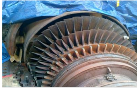
Gambar 6. Turbin Section PLTG Unit 4
