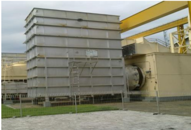
Gambar 3. Air Inlet Section PLTG Unit 4
