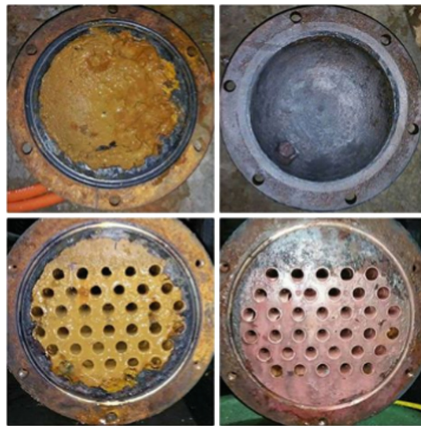
Fig. 6. Photo fouling During Commissioning ( Overhaul ) Earlier
