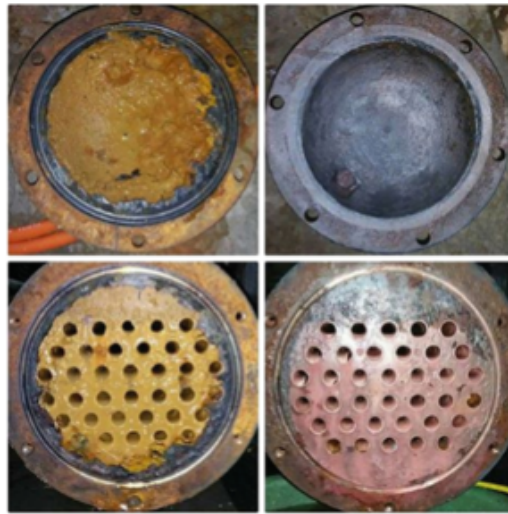
Fig. 6. Photo fouling During Commissioning (Overhaul) Earlier
