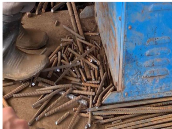
Fig. 1 Remaining Pieces of Steel Reinforcing
