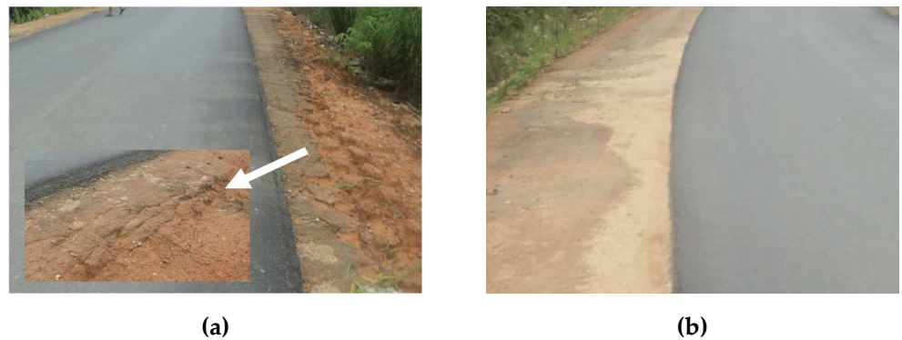
Figure 1. The appearance of soil-cement as a base (a) undergo wetting-drying cycles, and (b) non submerged road
