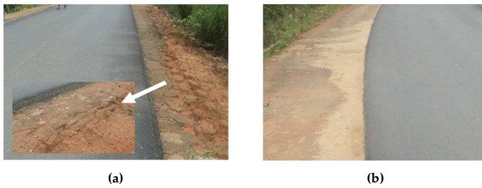
Figure 1. The appearance of soil-cement as a base (a) undergoing wetting-drying cycles, and (b) non-submerged road.
