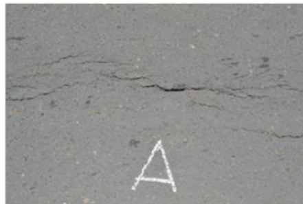
Figure 2 Road Surface Cracking Image
