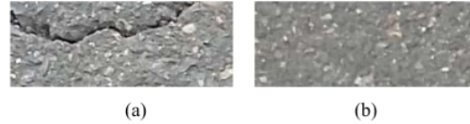
Fig.3 (a) With Crack (b) No Crack
