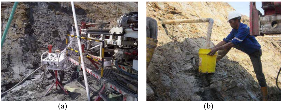
Figure 5. (a) Horizontal drilling process, and (b) installation of the perforated galvanized pipe
